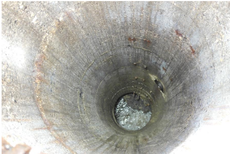
Cornish Lift Station Wet Well
